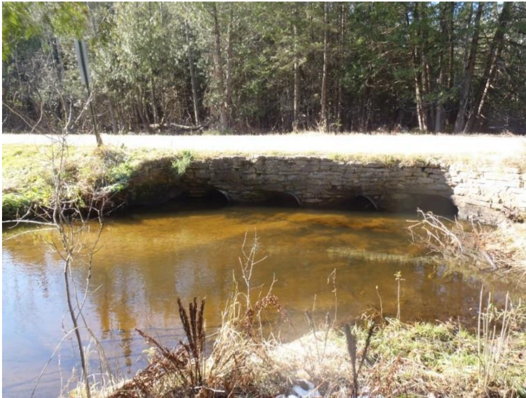
Current road/stream crossing structure on the North Branch Beaver Creek at 25 th Rd.
