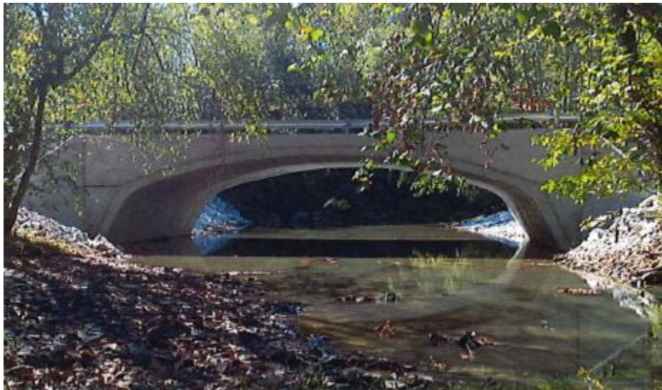
The proposed ecological culvert design will consist of a ConSpan bridge with poured footers and wing walls. The itemized budget for this proposed structure (below) was prepared by Trout Unlimited.
